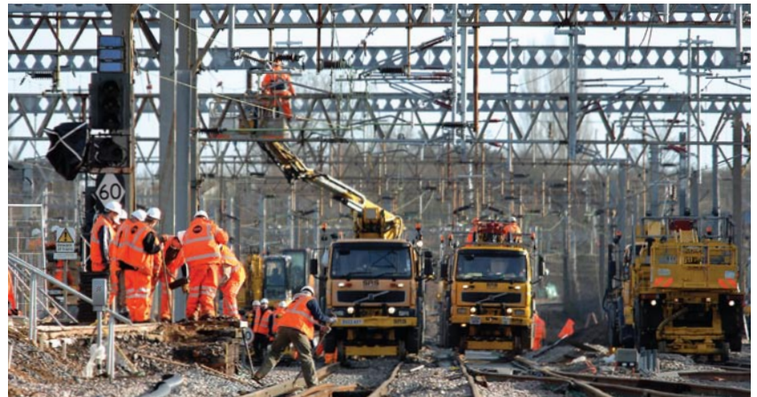
Asset renewal of overhead line equipment takes place at Rugby during the final stages of the massive West Coast Main Line modernisation project. Network Rail
